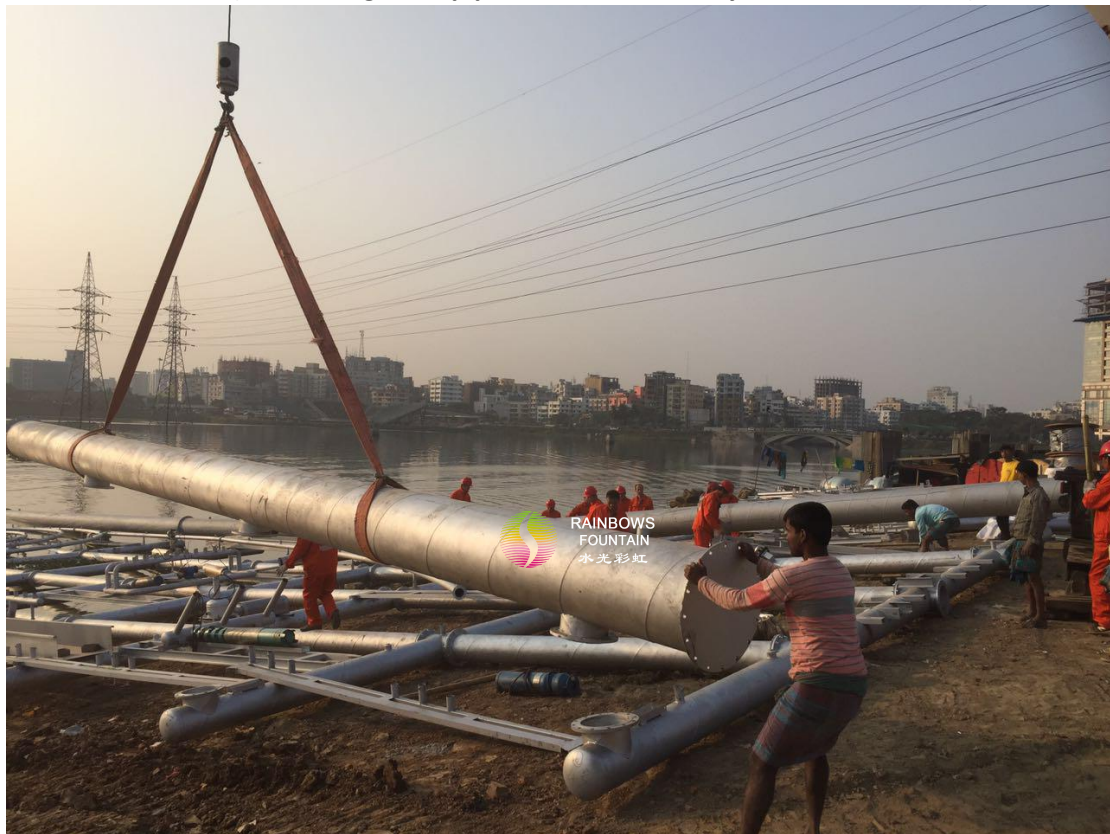
Installation on site(assembling main pipe on the shore firstly then move to lake)
